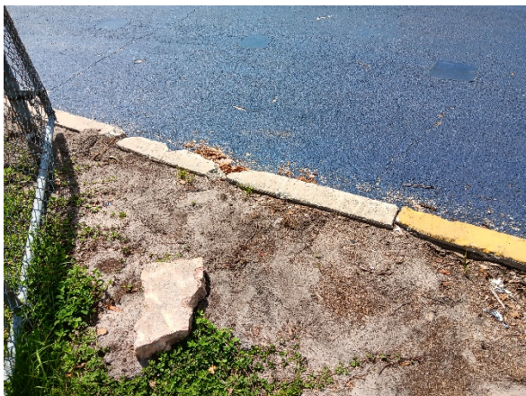
Existing curb damage near gate
