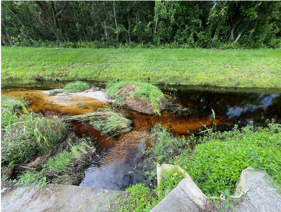
Figure 1 – Excess Silt within VWCD Canal – Received by CPH on December 31, 2024.
