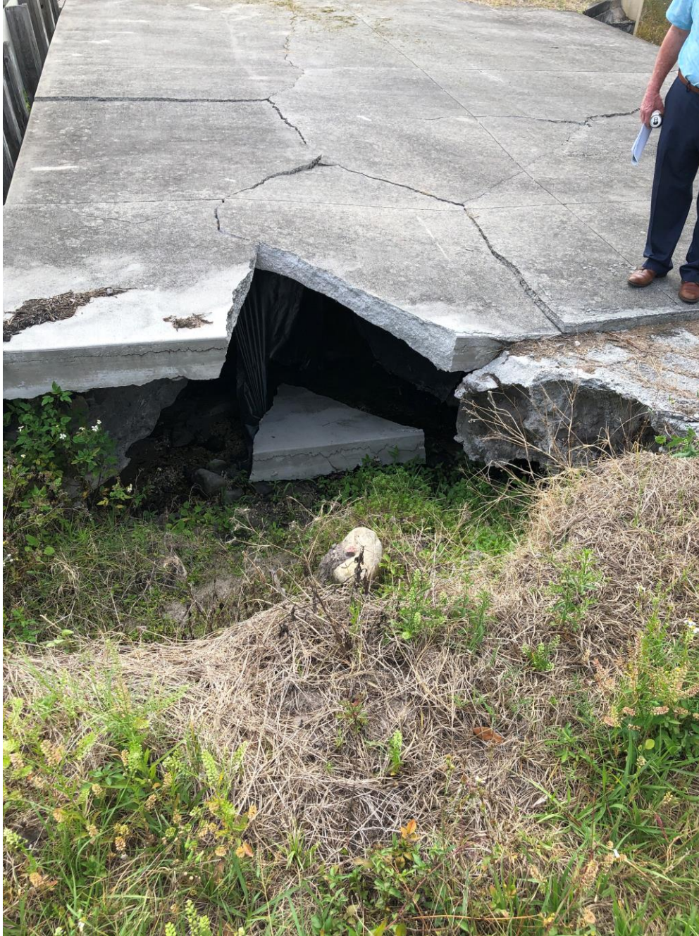
Figure 2 – Damage of outfall structure – Received by CPH on December 31, 2024.
