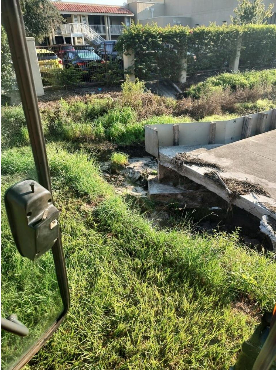
Figure 4 – Erosion of outfall structure – Received by CPH on December 31, 2024.
