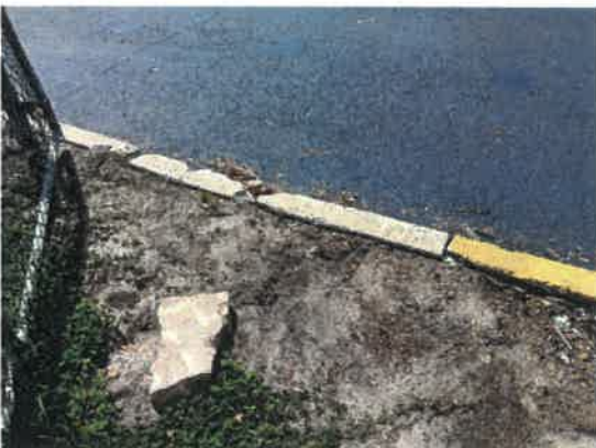
Existing curb damage near gate
